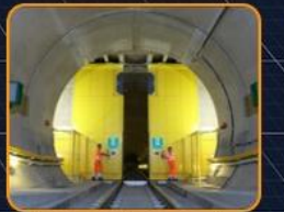
Emergency Doors and Gates
