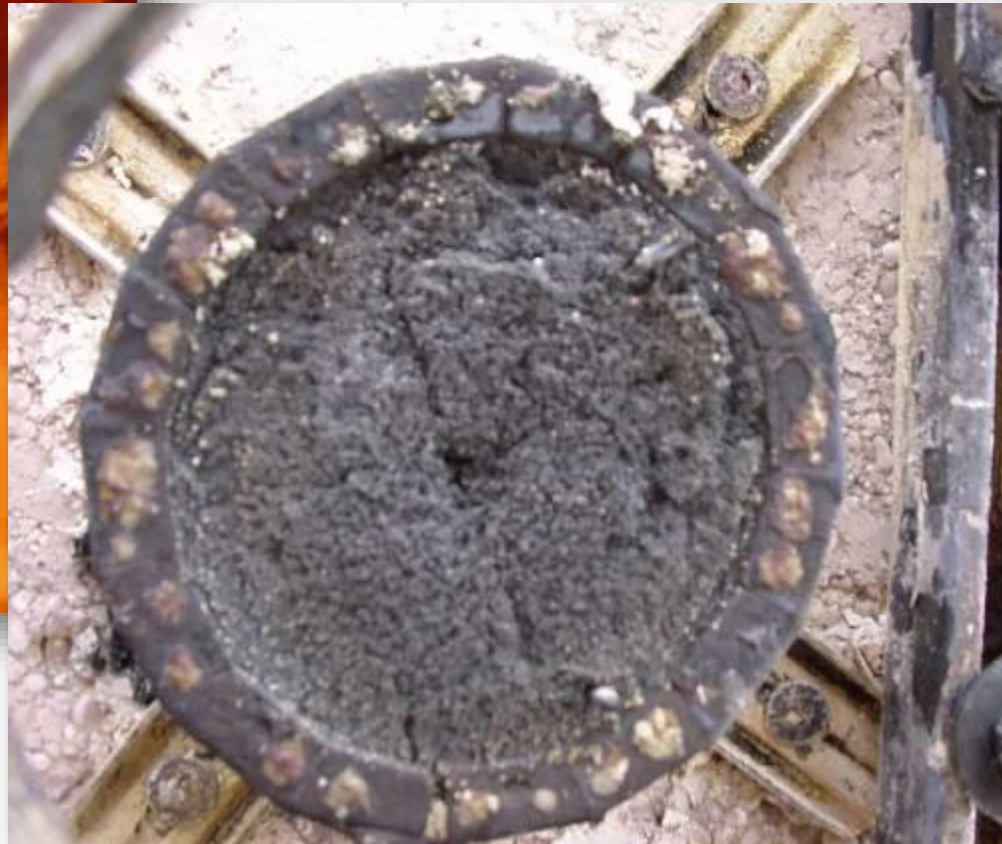
After fire exposure & hose stream
