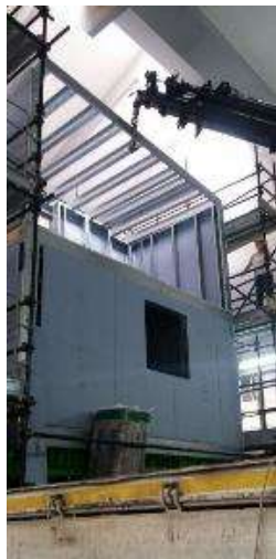
Walls and floors lifting
