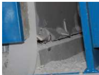
8. Collapse of panel-to-frame fixings
