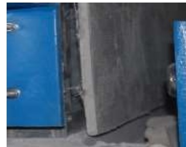
4. Detachment between walls and structural elements
