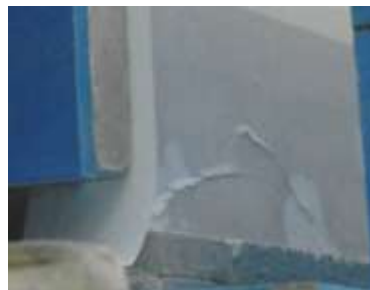
5. Cracks in the panels
