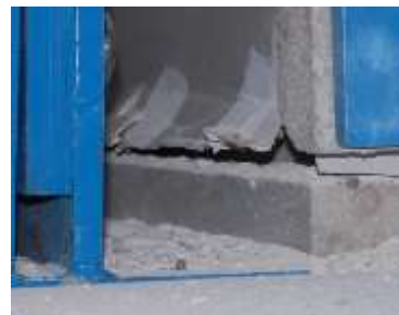
6. Corner crushing of panels
