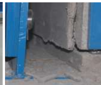
7. Crushing of exterior façade wall corner
